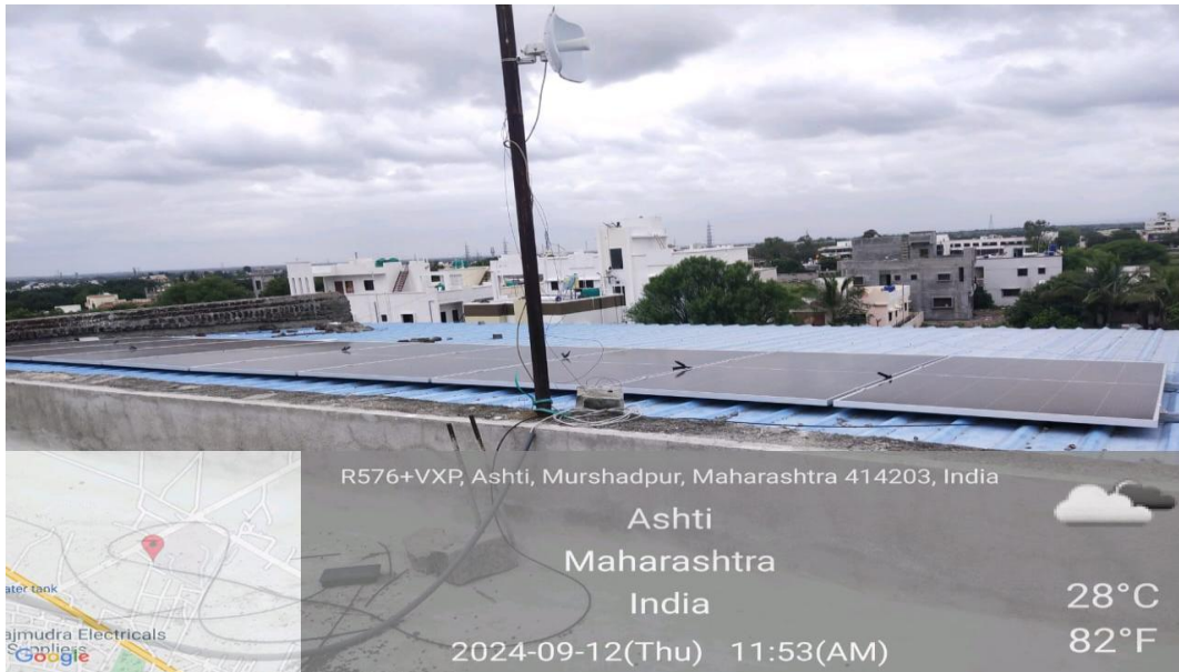
The college has installed a five kilowatt solar project for energy conservation.
