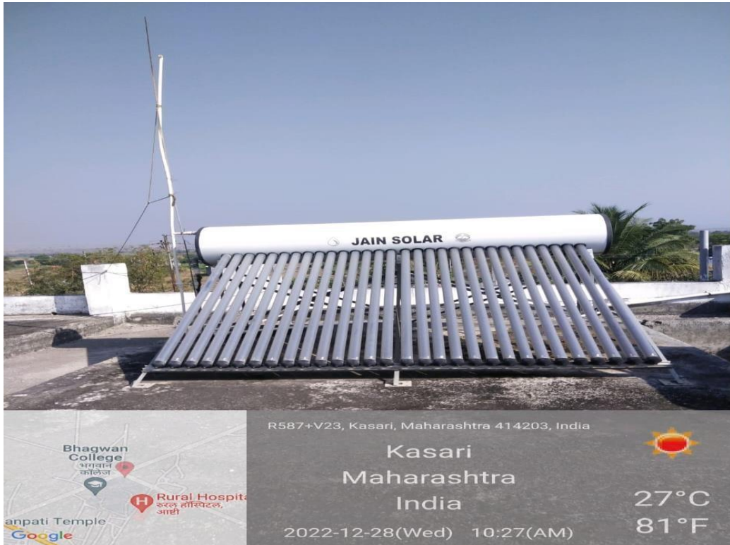
Use of Solar Energy/ Solar water Heater for Women's Hostel
